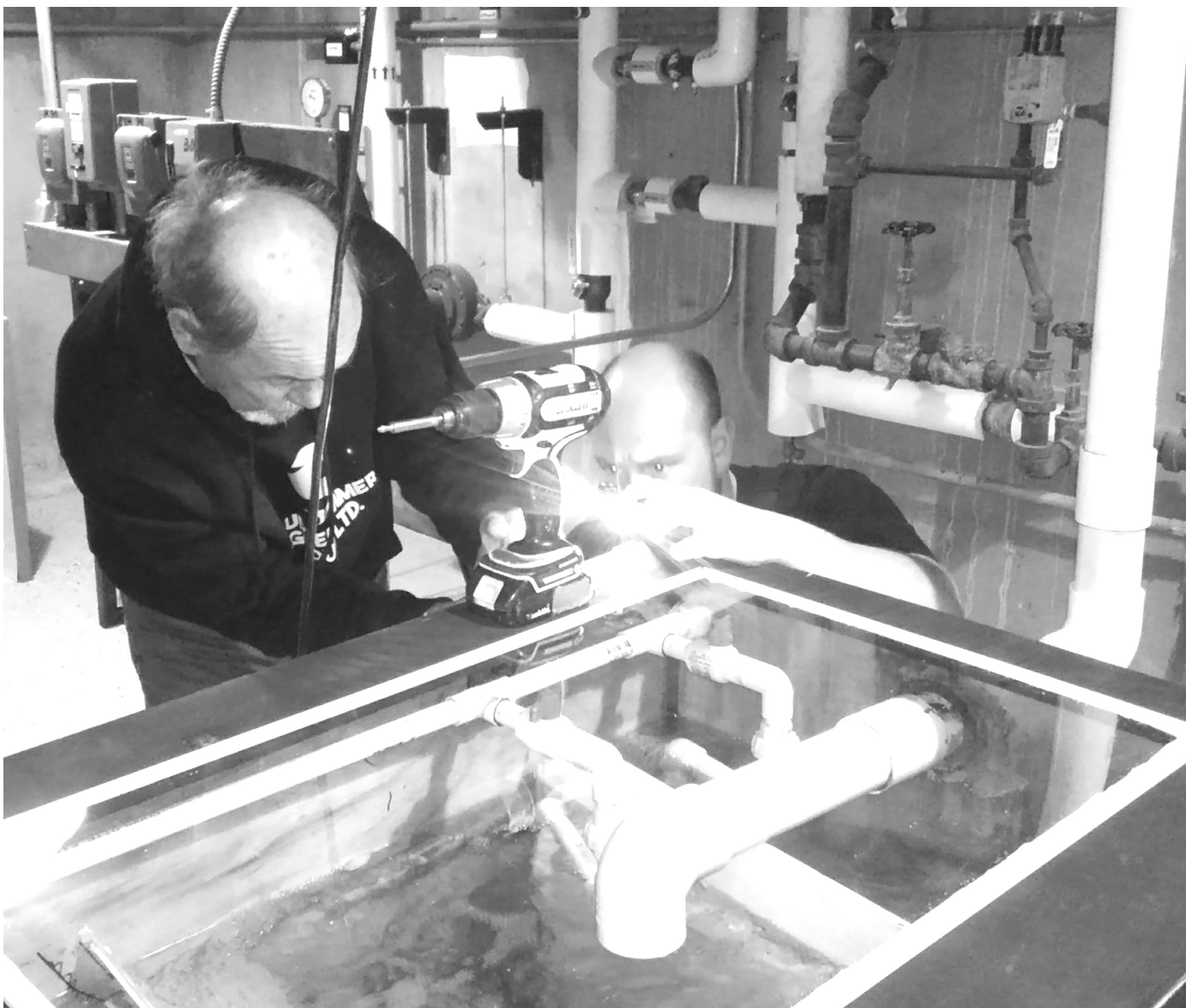
North Central Michigan College recently installed a small-scale waste-water treatment unit in the residence hall on the Petoskey campus. Courtesy photo
